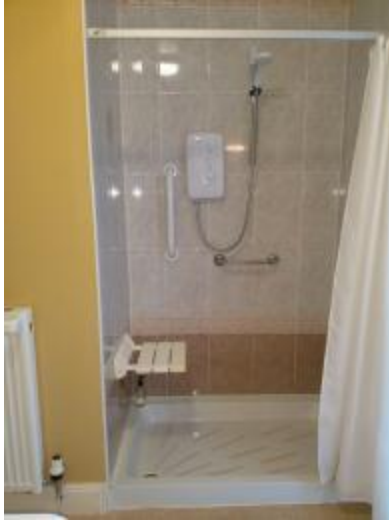
Ground floor bathroom shower showing flip seat lowered and two adjacent grab rails on shower wall
